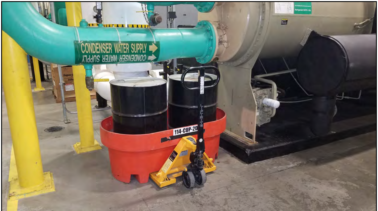
Drum Storage Area (114-CUP-2D) at Central Utility Plant - Building 114
