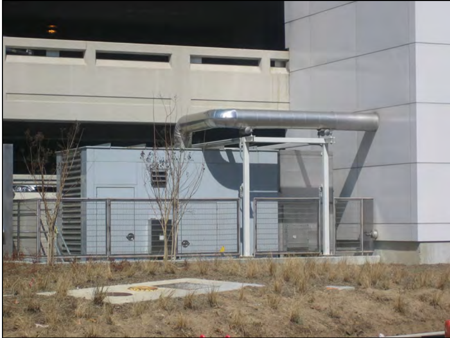
375-Gallon Diesel Fuel Emergency Generator Sub-Base Tank (160-HPG-2A) By Terminal Loop below Skywalk
