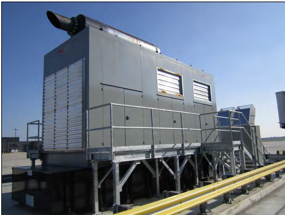
3540-Gallon Diesel Fuel Emergency Generator Sub-Base Tank (C-3A) At Pier C (Between Gate C-7 and C-Tower)
