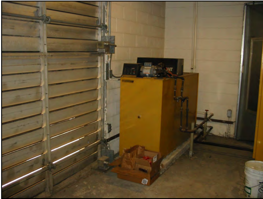
275-Gallon Diesel Fuel Emergency Generator Day Tank (101-FLV-1A) Inside Field Lighting Vault (Building 101)
