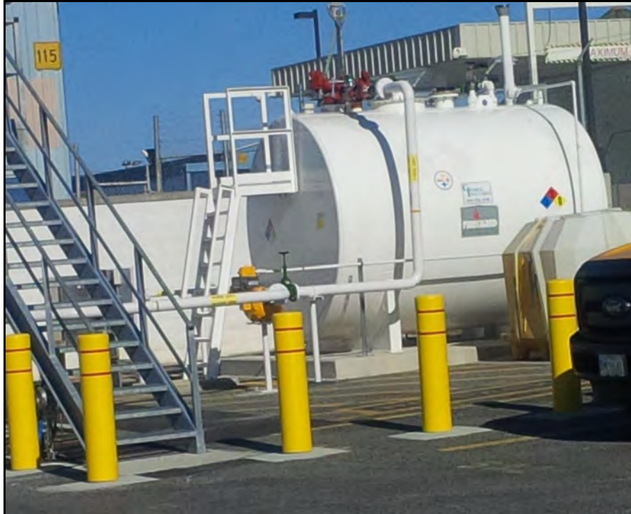
4000-Gallon Diesel Fuel Tank (116-FM-4A) Behind Field Maintenance Building
