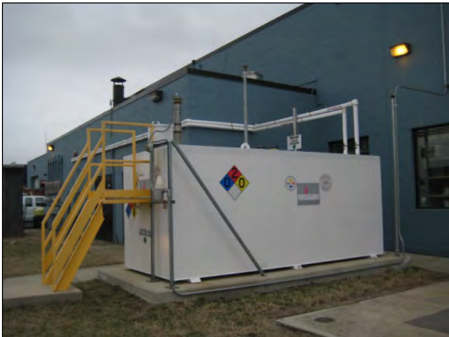
3,000-Gallon No. 2 Fuel Oil Tank (123-PS-1A) Outside Old Paint Shop (Building 123)
