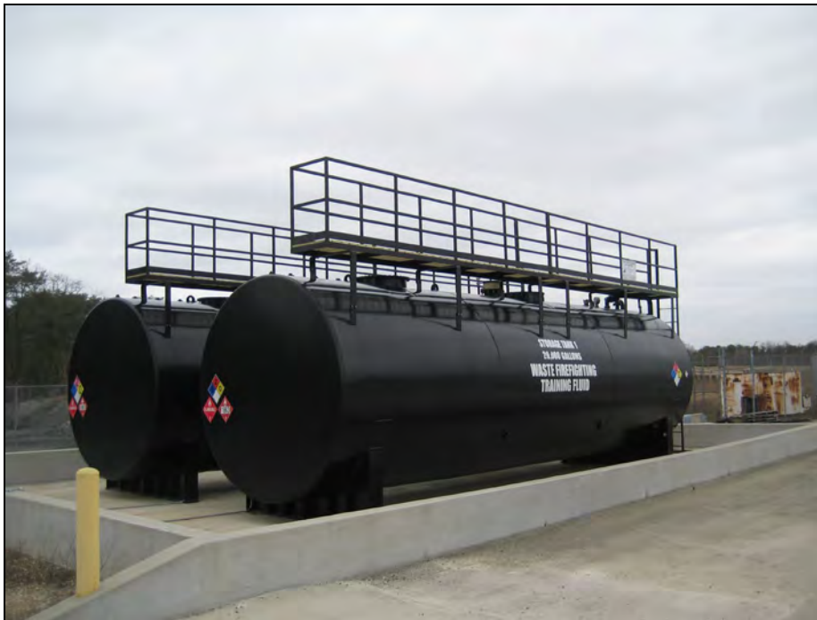
20,000-Gallon Jet A / Diesel Fuel / Firefighting Foam / Water Mixture Tanks (FTF-3A and FTF-4A) At Fire Training Facility
