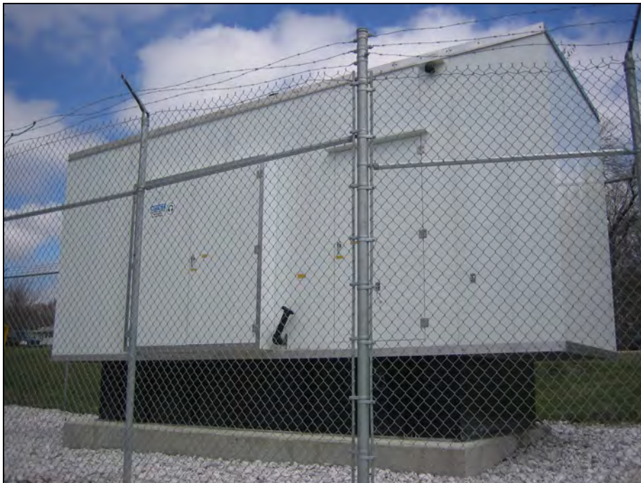
700-Gallon Diesel Fuel Emergency Generator Sub-Base Tank (172-MAC-1A) By MAA Radio Tower Outside MAC Building (Building 172)
