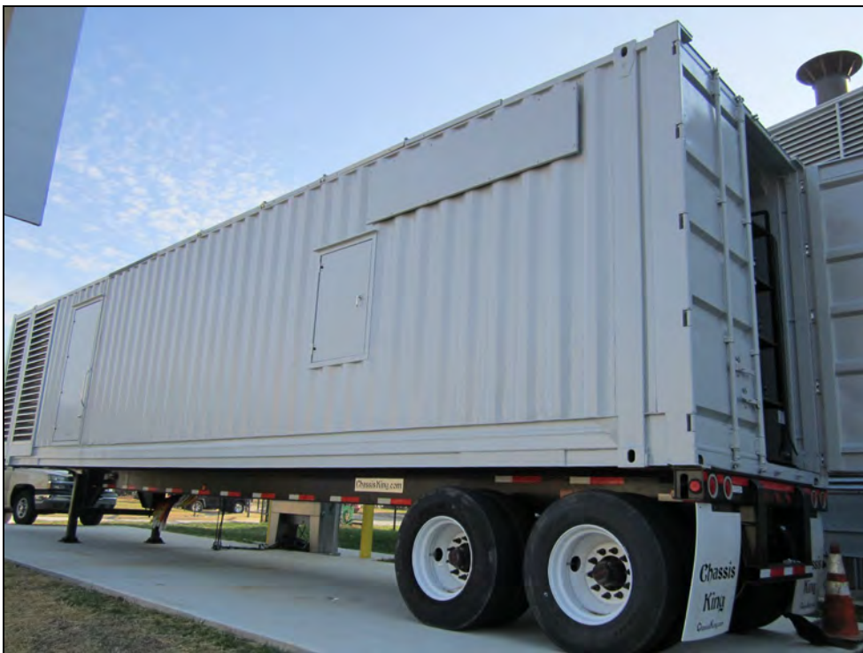
2800-Gallon Diesel Fuel Portable Emergency Generator (114-CUP-1M) Normally Parked At Central Utility Plant - Building 114
