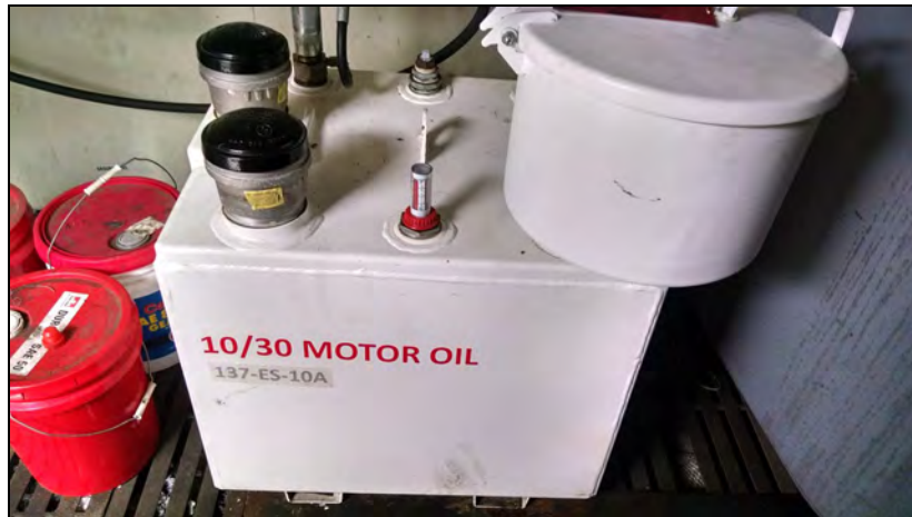
60-Gallon Tank for Motor Oil (137-ES-10A) Inside Shed behind Heavy Equipment Shop (Building 137)
