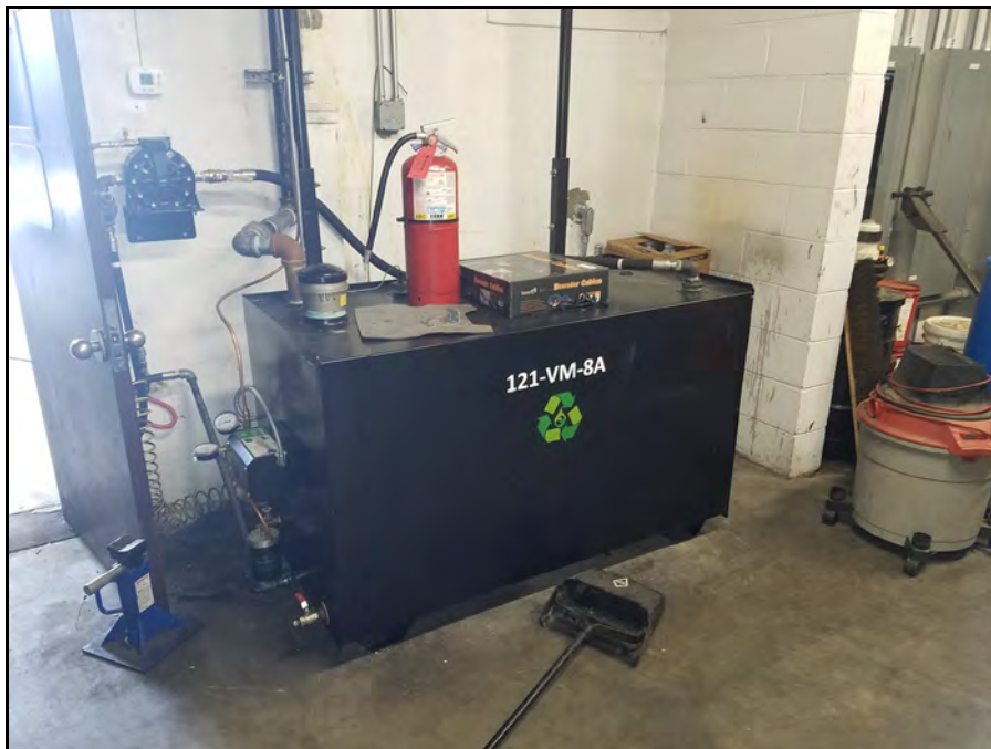
250-Gallon Heating Oil Tank (121-VM-8A) Inside Room 121-13 of Vehicle Maintenance Shop (Building 121)
