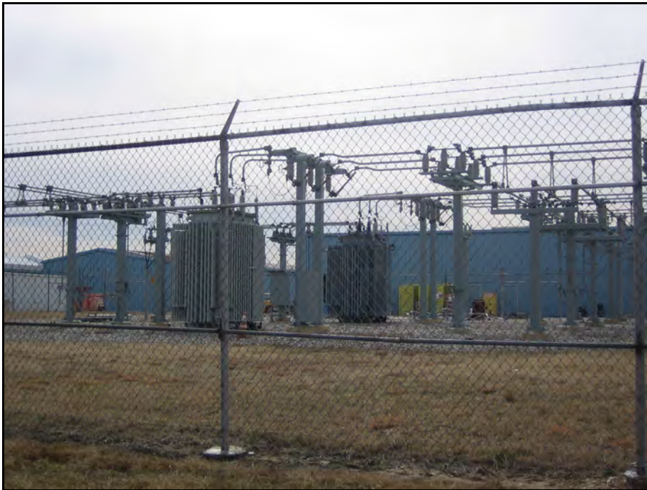
Transformers at Old North Substation (ONS-1T, ONS-2T)
