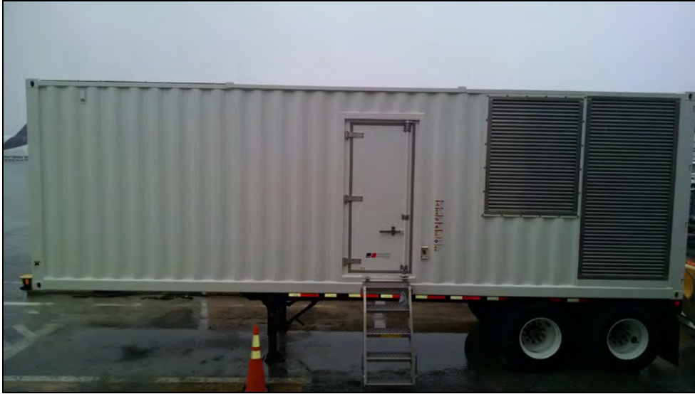
1,200-Gallon (MOBILE-4M) Diesel Fuel Emergency Portable Generator Normally Parked Behind Cargo Building 112
