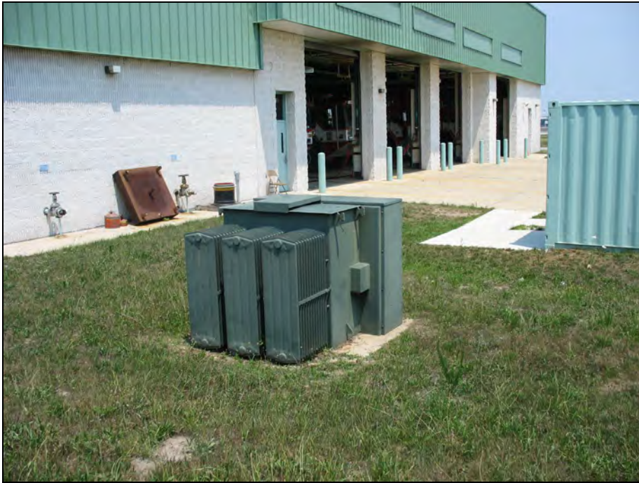
Transformer at Aircraft Rescue and Firefighting Facility (105-ARFF-1T)
