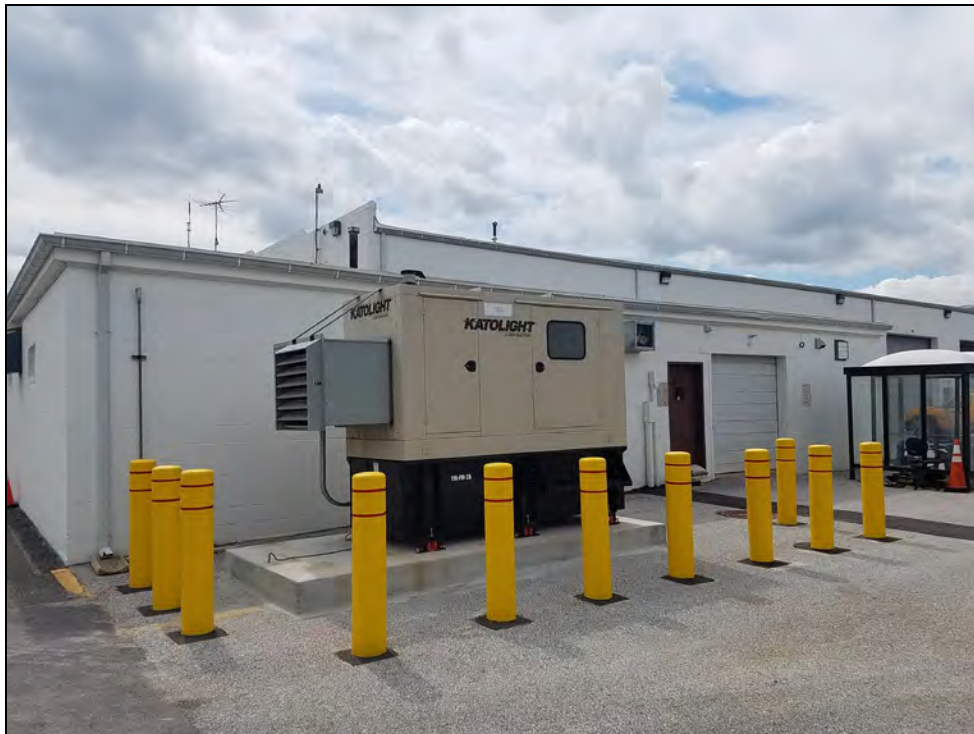
375-Gallon Diesel Fuel Emergency Generator Sub-Base Tank (116-FM-2A) Outside at Field Maintenance (behind Building 116)
