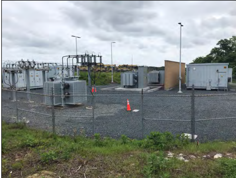
Transformers at South Substation (SS-1T, SS-2T, SS-3T)
