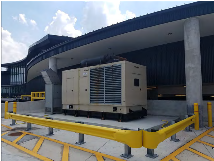
660-Gallon Diesel Fuel Emergency Generator Sub-Base Tank (E-1A) At Pier E - International Terminal (public side of terminal)
