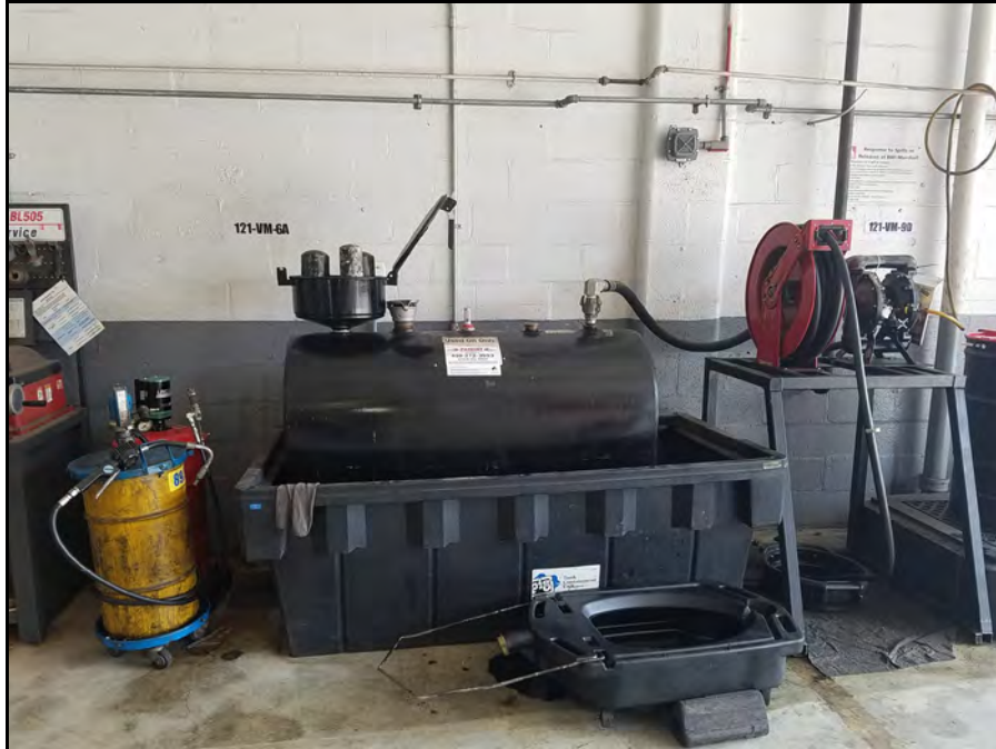
275-Gallon Used Oil Tank (121-VM-6A) Inside Vehicle Maintenance Shop (Building 121)
