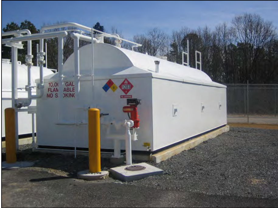
10,000-Gallon Jet A / Diesel Fuel Mixture Tank (FTF-2A) At Fire Training Facility
