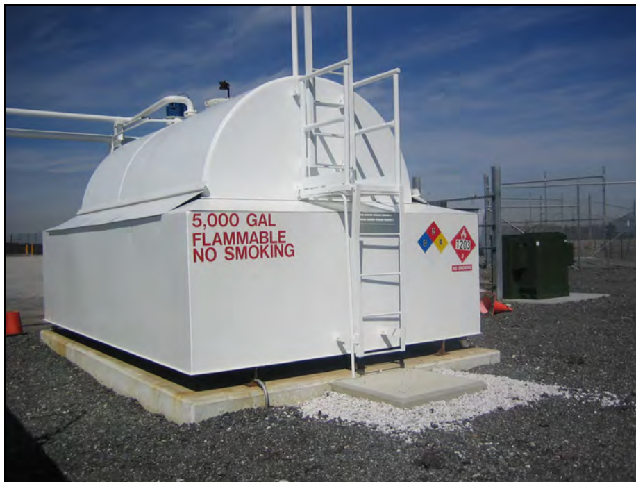
5,000-Gallon Jet A / Diesel Fuel Mixture Tank (FTF-1A) At Fire Training Facility
