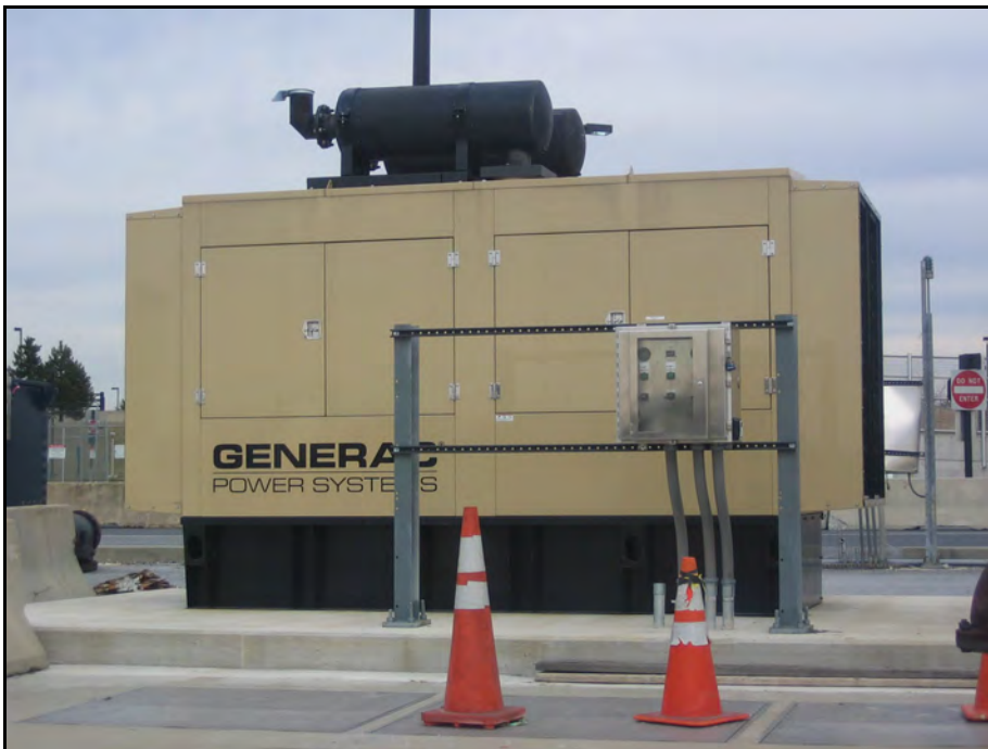
430-Gallon Diesel Fuel Emergency Generator Sub-Base Tank (A-2A) Adjacent to Taxiway A by Triturator
