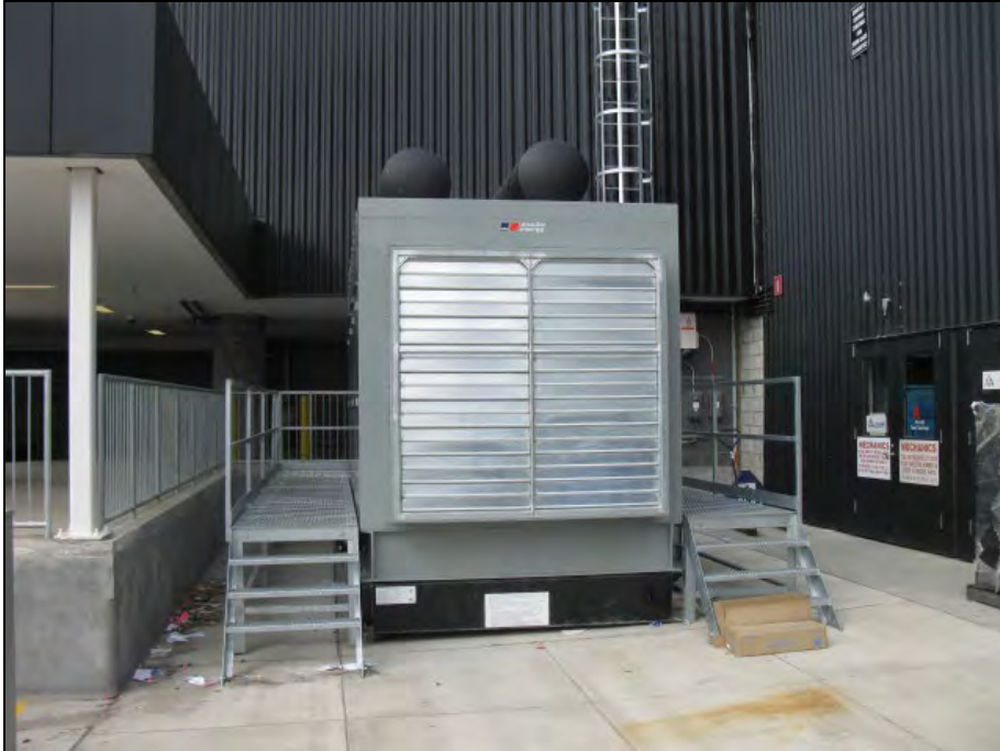
800-Gallon Diesel Fuel Emergency Generator Sub-Base Tank (C-4A) At Pier C (Gate C-4)
