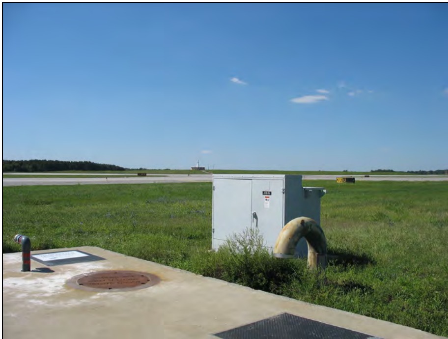
Transformer at 28 Pump Station (28PS-1T)
