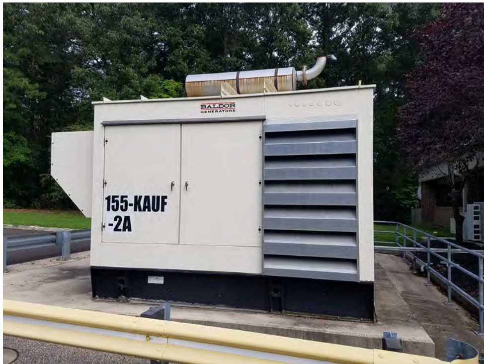
411-Gallon Diesel Fuel Emergency Generator Sub-Base Tank (155-KAUF-2A) Outside Kauffman Building (Building 155)
