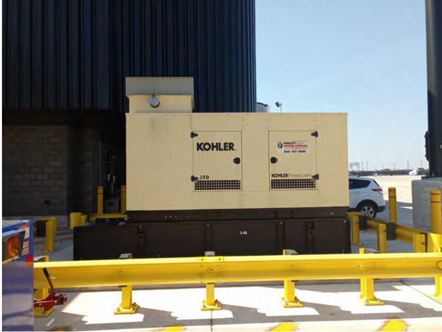
555-Gallon Diesel Fuel Emergency Generator Sub-Base Tank (E-4A) At Pier E - International Terminal (between Gates E-5 & E-7)
