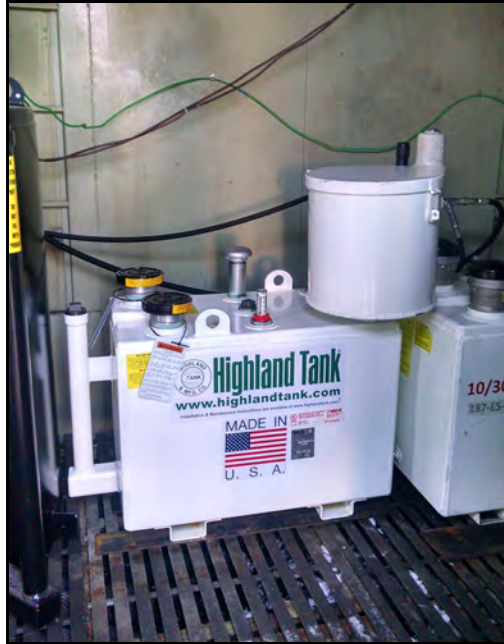
60-Gallon Tank for Motor Oil (137-ES-11A) Inside Shed behind Heavy Equipment Shop (Building 137)
