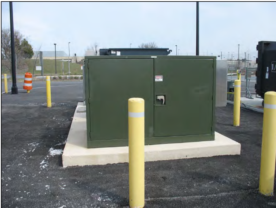
Transformer at Triturator Facility (TRI-1T)
