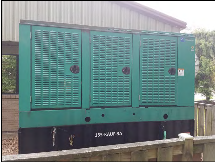
310-Gallon Diesel Fuel Emergency Generator Sub-Base Tank (155-KAUF-3A) Outside Kauffman Building (Building 155)
