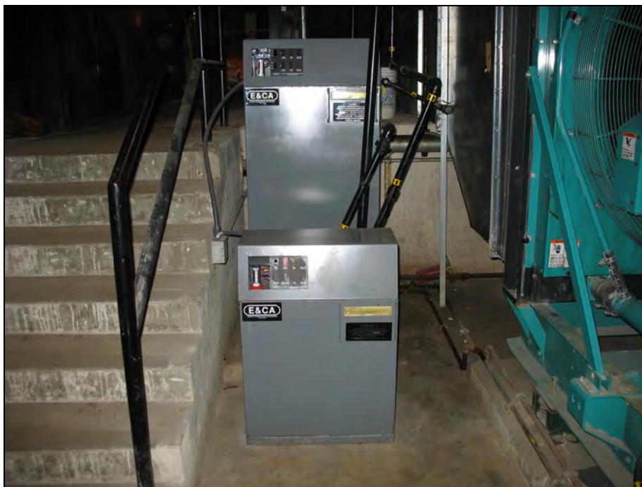
200-Gallon Diesel Fuel Emergency Generator Day Tank (160-HPG-1A) Inside Hourly Parking Garage (Building 160)
