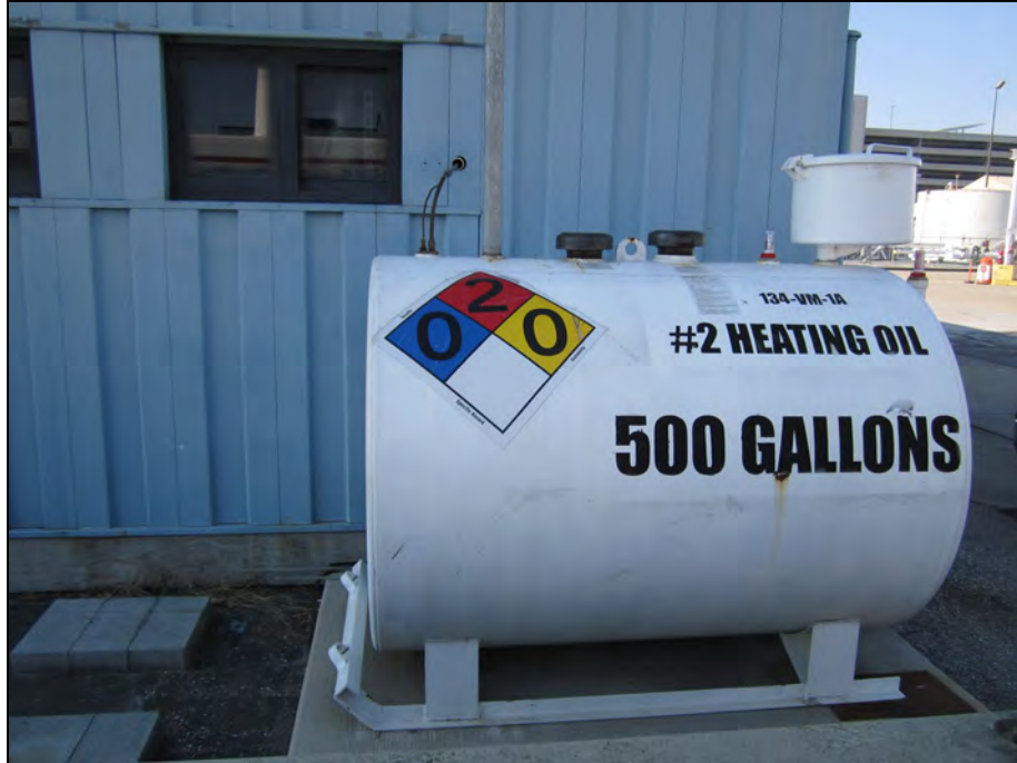
500-Gallon Heating Oil Tank (134-VM-1A) Outside Vehicle Maintenance (Building 134)
