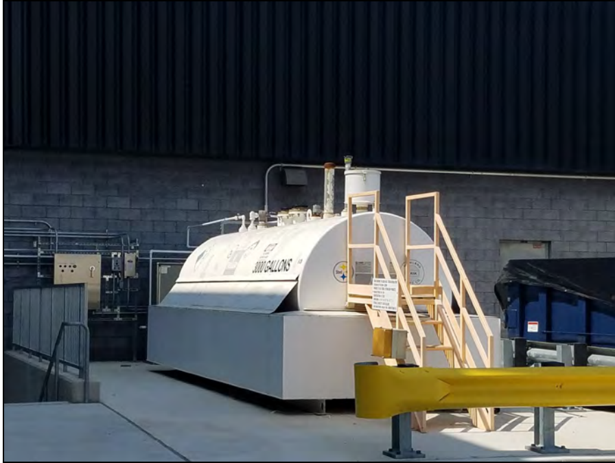
3,000-Gallon Diesel Fuel Supply Tank (E-2A) to Emergency Generator Day Tank E-3A at Pier E (International Terminal)
