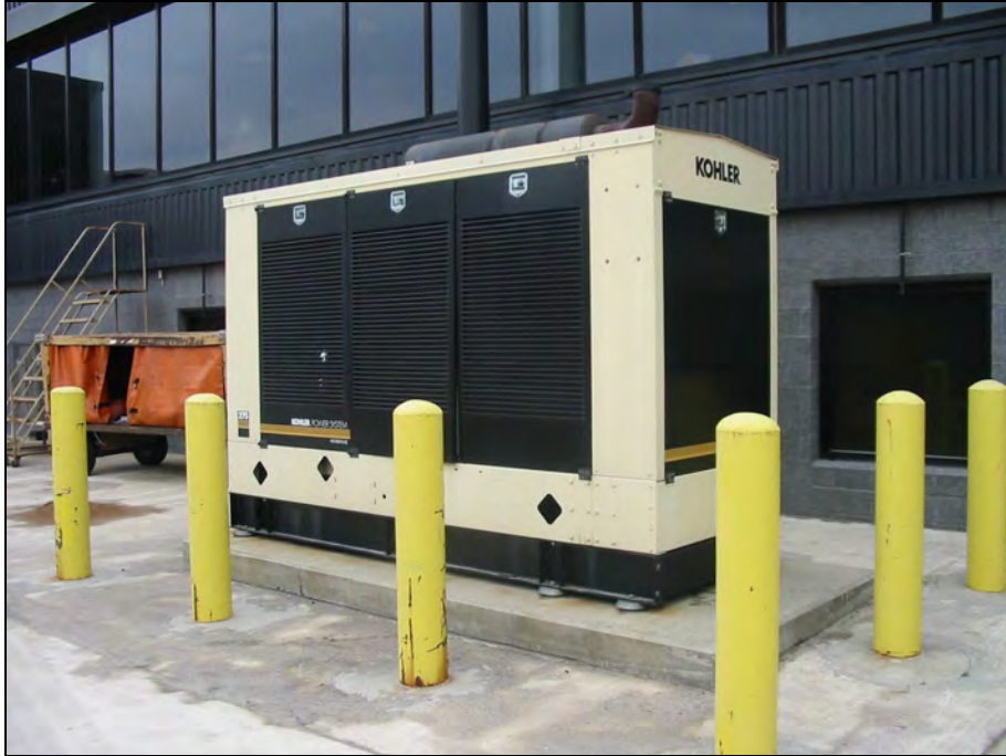
150-Gallon Diesel Fuel Emergency Generator Sub-Base Tank (B-1A) At Pier B (Domestic Terminal)
