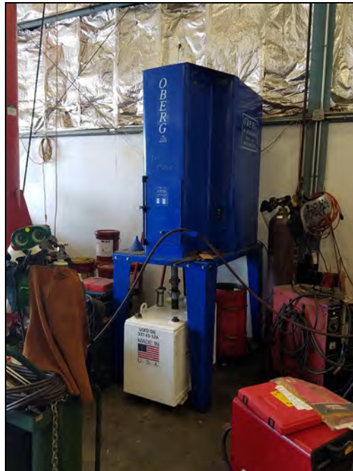
60-Gallon Tank for Used Oil from Drained Filters (137-ES-12A) Heavy Equipment Shop (Building 137)
