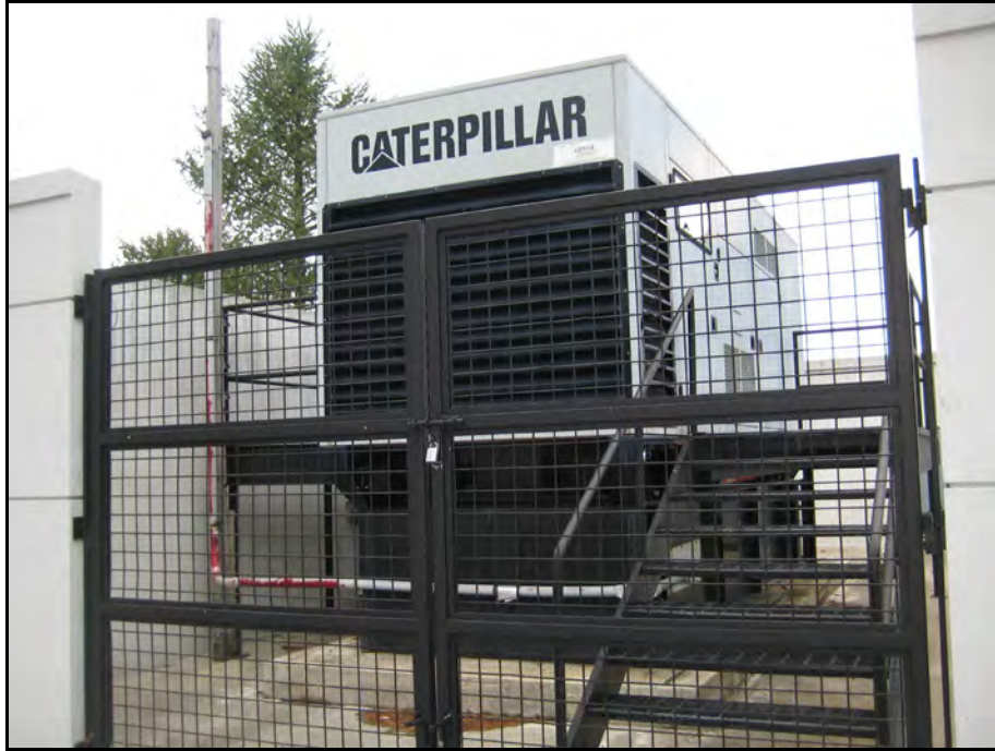
1,750-Gallon Diesel Fuel Emergency Generator Sub-Base Tank (140-DPG-1A) Outside Daily Parking Garage
