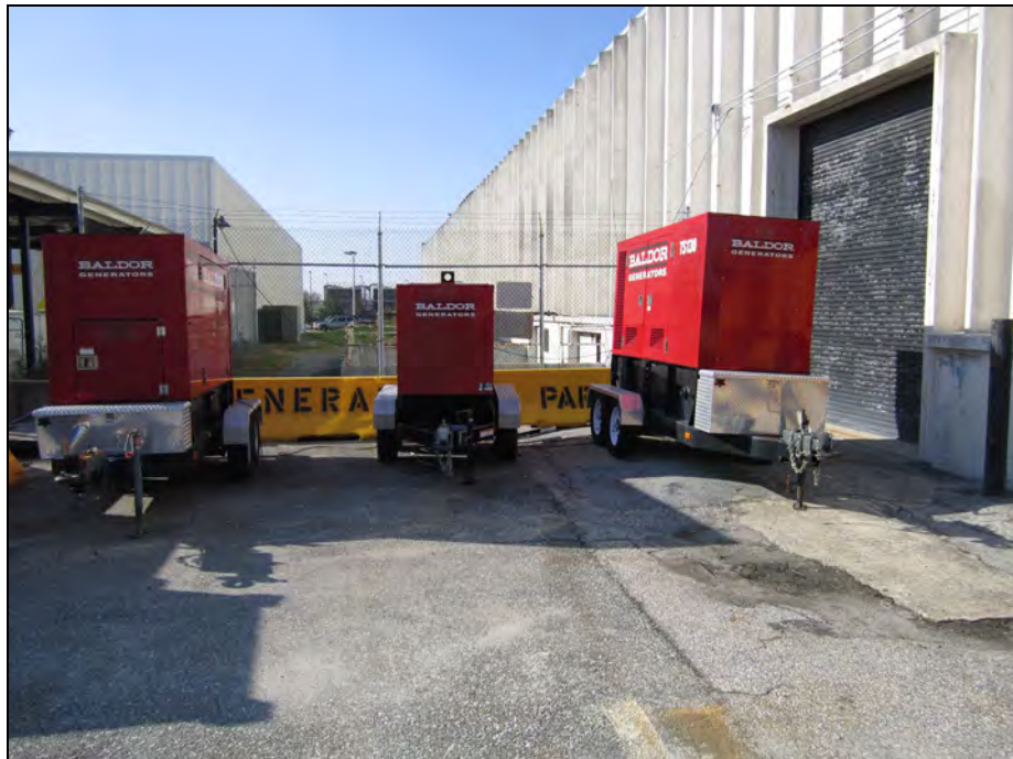
100-Gallon (MOBILE-1M), 160-Gallon (MOBILE-2M), and 80-Gallon (MOBILE-3M) Diesel Fuel Emergency Portable Generators Normally Parked At Cargo (air side) between Building 112 and Building 113
