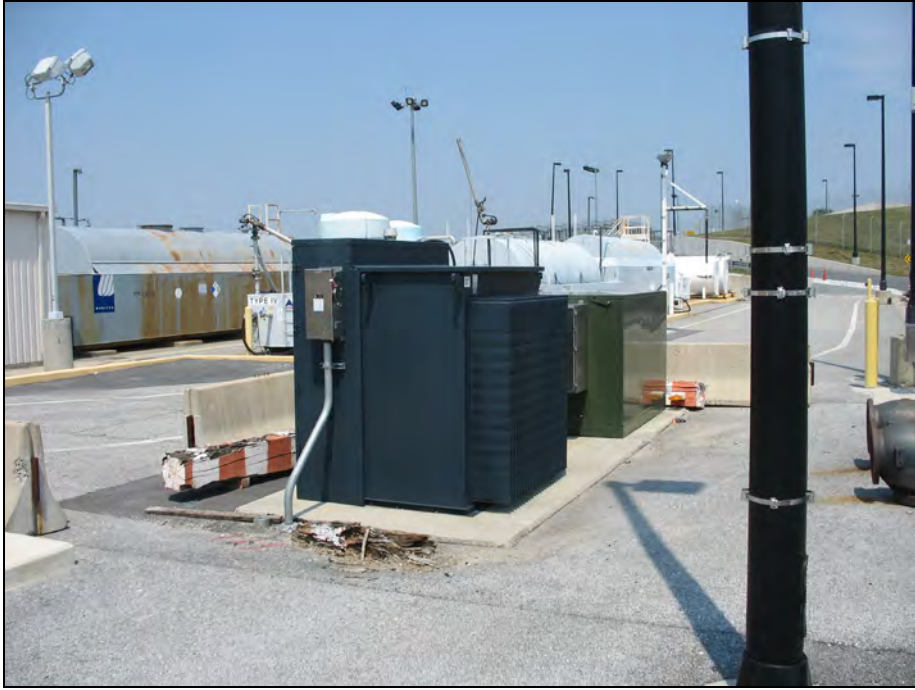
Transformer at Glycol Facility (GLY-1T)
